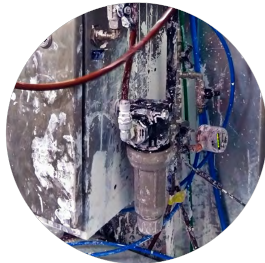
Contamination of surrounding during manual filter maintenance after a period of 6 months
